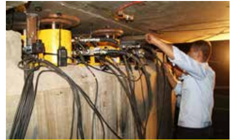
HYDRARITE General Purpose Cylinders with tilt saddles are lifting the bridge deck in pier reconstruction.
